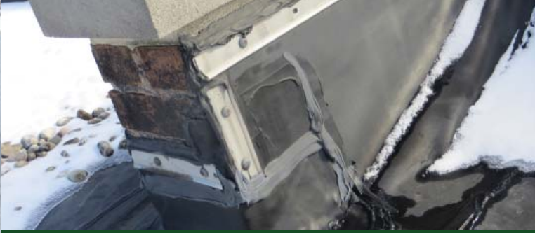
The library's existing roof is at end of its expected life and has already undergone several repairs and patch jobs.
